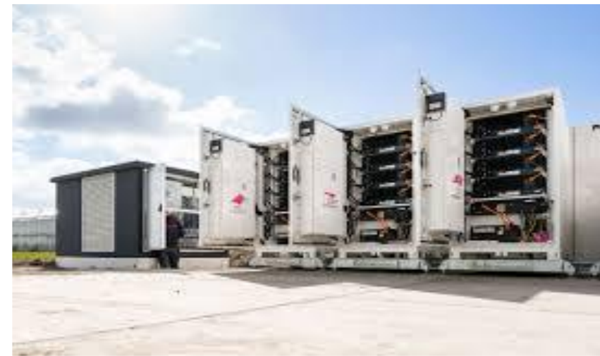
DYNAMIC BATTERY SYSTEMS
