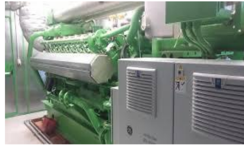
COMB. HEAT & POWER UNIT
